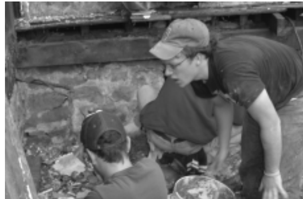
At left: With the demo complete, the guys had to get down and dirty on the foundation.
